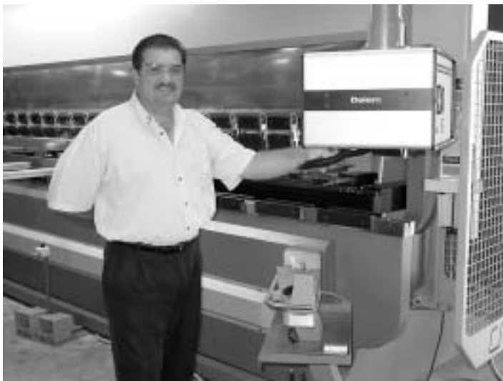
Rodney Bohner with the assembled, ready-to-run brake press in the Mickey machine room in High Point, NC
