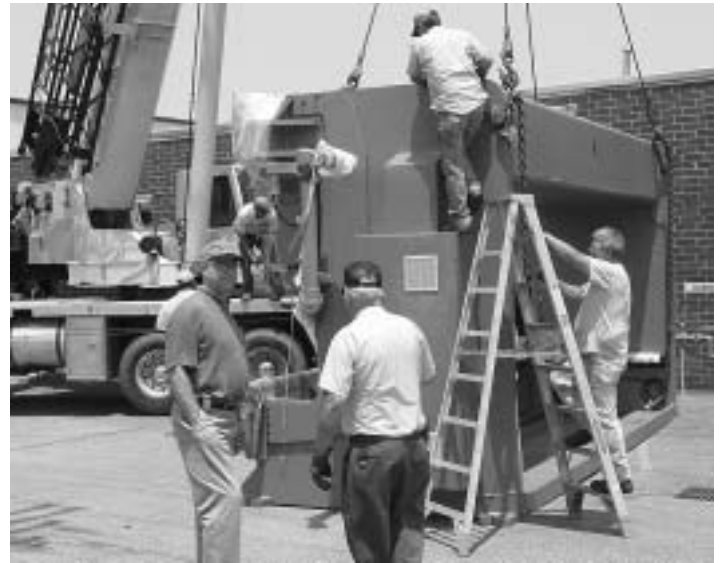
Joe Godwin, Project Manager for Guy M. Turner, Inc., moving engineers (facing camera), oversees the unloading and technical preparation for moving the sub assemblies of the CR Electronics' brake press into Mickey's 17,000-square-foot machine room.
